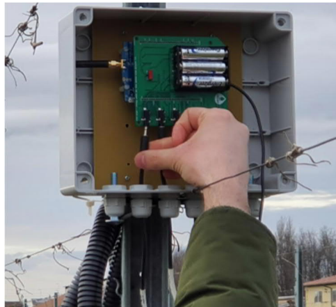
FIGURE 2. UNIBO SOIL PROBE SENSOR.
